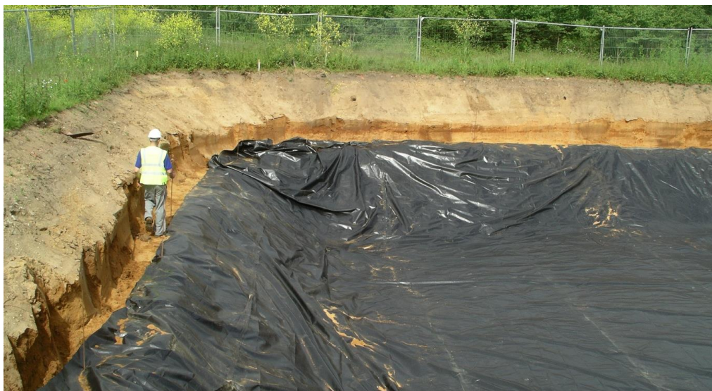
Battered sides (beneath barrier) and step batter at 2 m depth to facilitate safe installation of root barrier.
