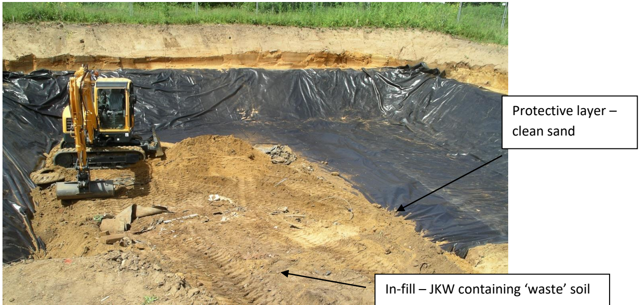
Placing a layer of soil across the base of a burial cell.
