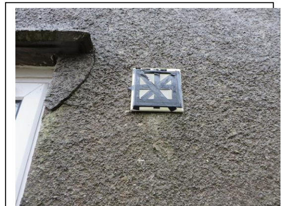
Fig 6. An example of an intermittent fan which had been covered by the occupant. In many instances the alterations may not be so obvious.
