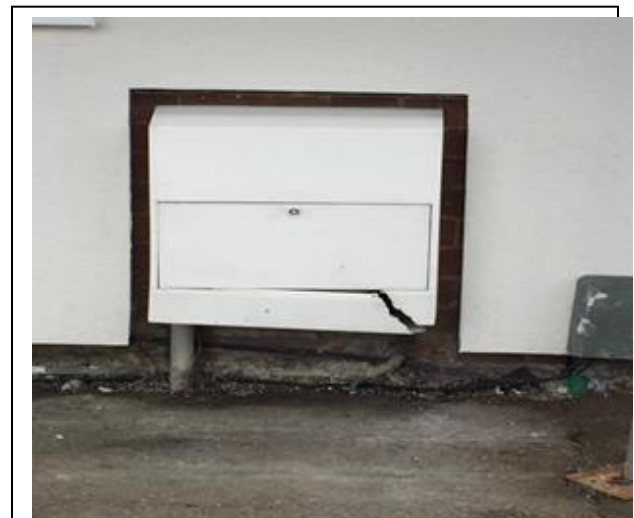
Fig 2. Another example of discontinuous insulation which will result in temperature differentials in the structure and may result in condensation and mould growth problems.
