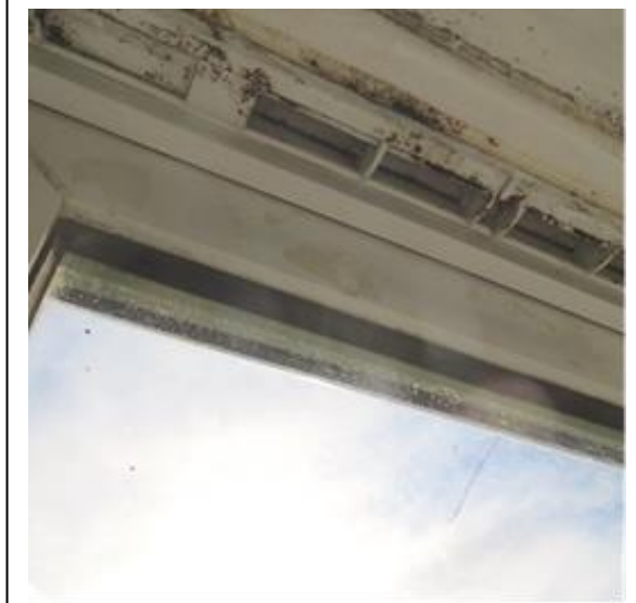
Fig 7. The picture above shows a trickle vent which was stuck to the window frame but without sufficient opening.
