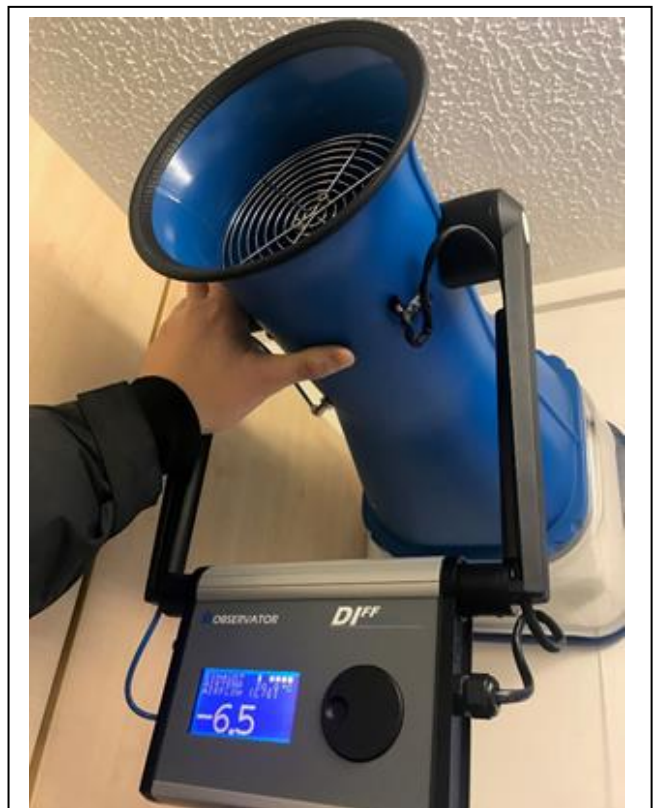
Fig 8. Unconditional method of testing a type 1 ventilation system using a powered hood.
